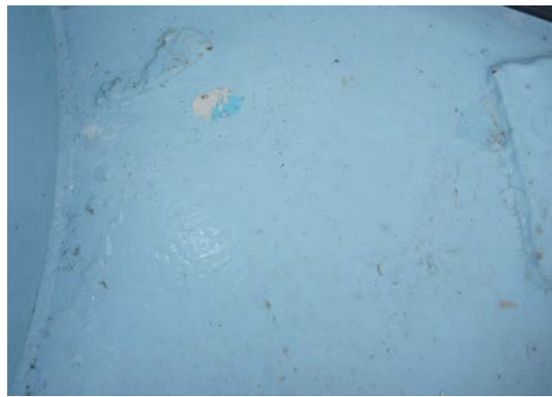
Spot Failure and Mud Cracking on the Roof
